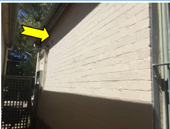
Photo 5. Exterior, ground level, throughout, walls – lead-containing cream upper paint system.
